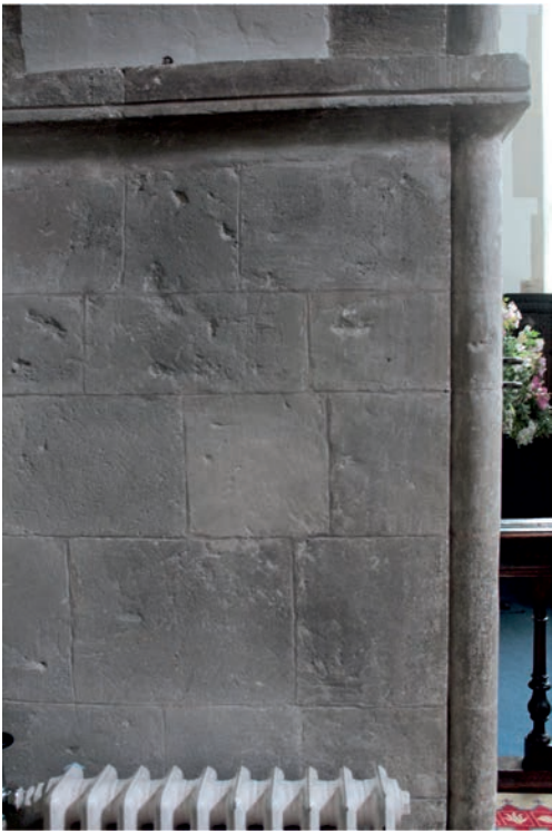
27 - Above, the return wall at the west end of the north chapel south wall. Feint traces of fictive masonry line decoration remain here.
