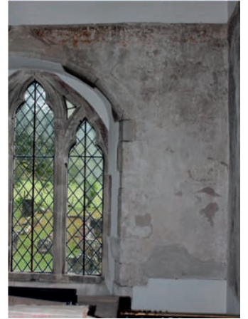
16 - Below, detail from 15 showing painted decoration from both the C14 and the later scheme (C15 or early C16?). The condition of the plaster in this area is poor, there is much detachment. Evidence for the detachment can be seen in the number of cracks in the plaster. Please also see illustration 3.
