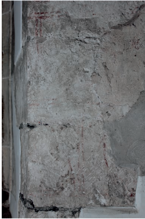
13 - Far left, area of replastering carried out before the C14 scheme was applied. See illustration 4.
